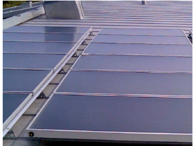
Figure 2.18 Solar panels on the University's roof.
